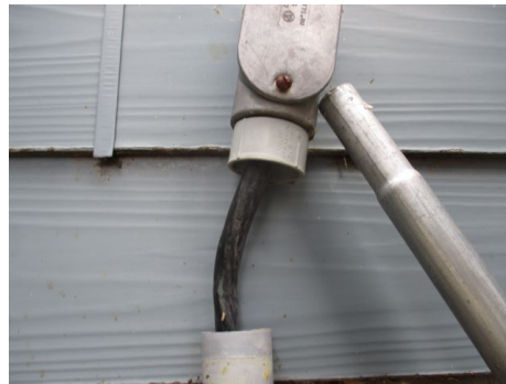
Settled conduit on wiring by patio
