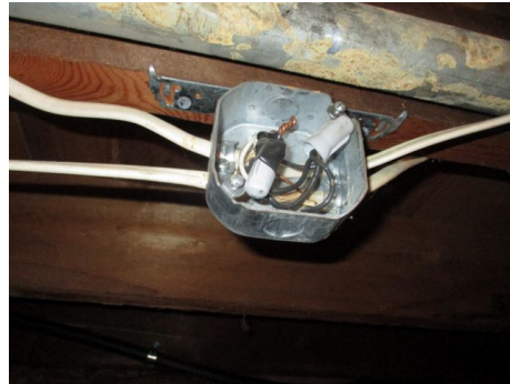
Open junction boxes in basement
