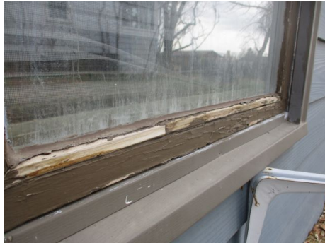
Weathered wood & peeling paint on windows & trim
