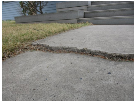
Raised concrete on front sidewalk
