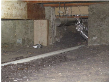
Dryer vented to basement
