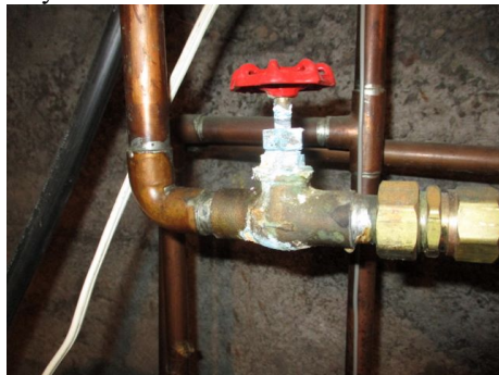
Corrosion on water lines in basement
