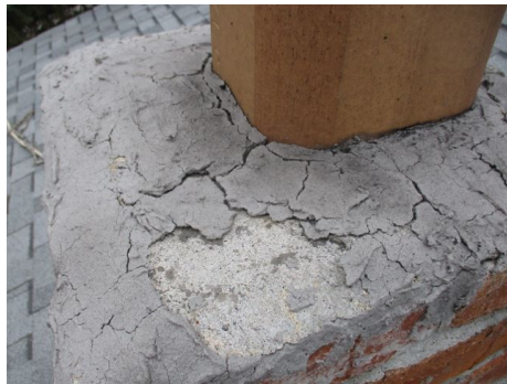
Loose/cracked mortar on chimney top
