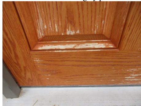
Weathering on front door
