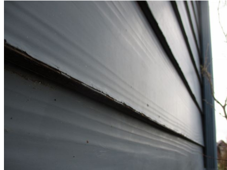
Weathered edges on siding
