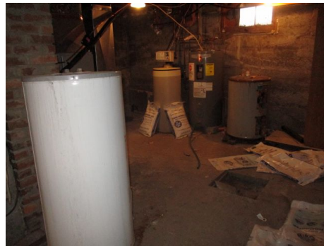
Several old water heaters in basement
