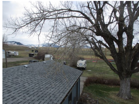
Tree branches hanging over roof
