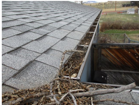
Gutters need cleaning
