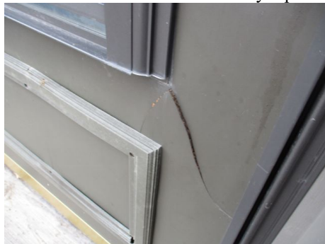
Damaged/deterioration on storm door
