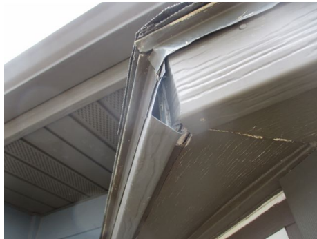
Loose fascia metal by front windows
